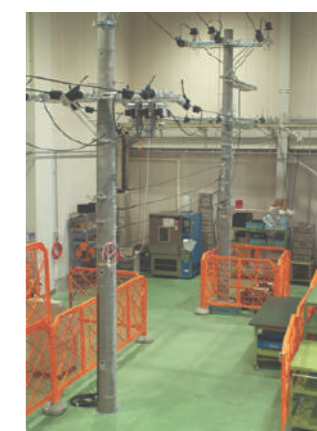
Simulated power pole for electricity distribution line
